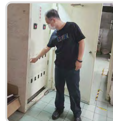
Emergency Power Shutoff
