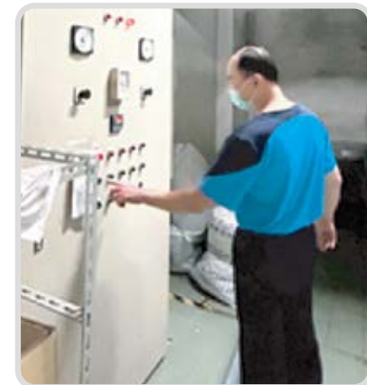
Emergency Power Shutoff
